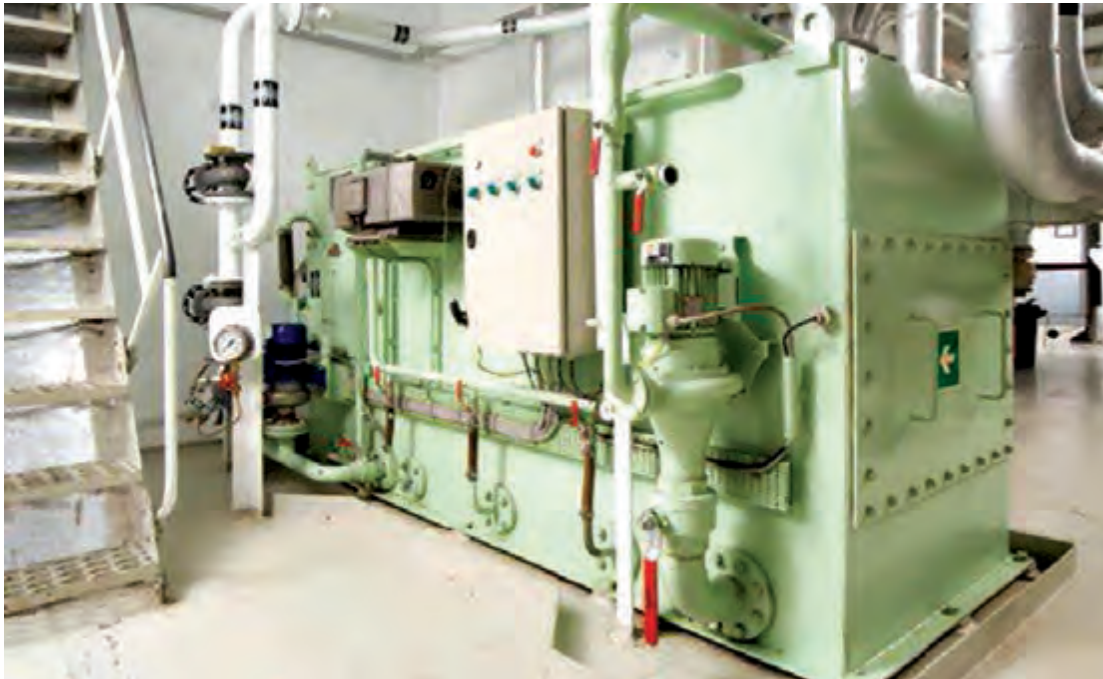
sewage treatment plant
