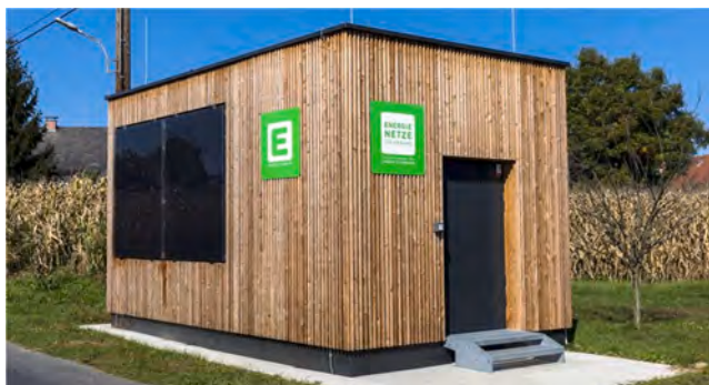
Fig. 9. Community battery located at the Heimschuh pilot site in Styria, Austria.
