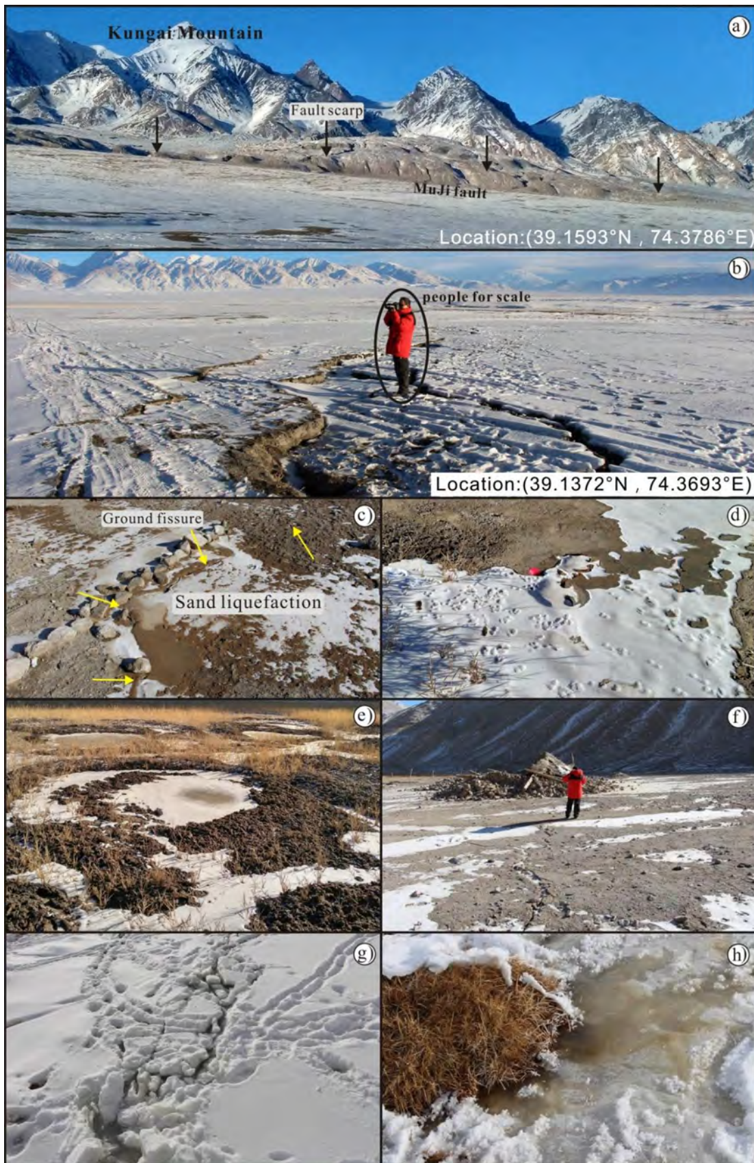
Fig. 10. Field photographs of this earthquake. (a) The fault scarp of the Muji fault. (b) Coseismic ground fissures in the Bulake study area. (c) and (d) Liquefaction originating from ground fissures in the epicenter. (e) The primary spring at the epicenter. (f) Property damage caused by coseismic ground fissures. (g) and (h) Sand liquefaction in the Bulake study area.
