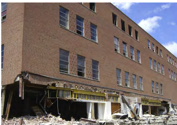
Fig. 15. Ohio Union Building used for testing by Song and Sezen [215]. Photo by courtesy of Halil Sezen (Ohio State University).
