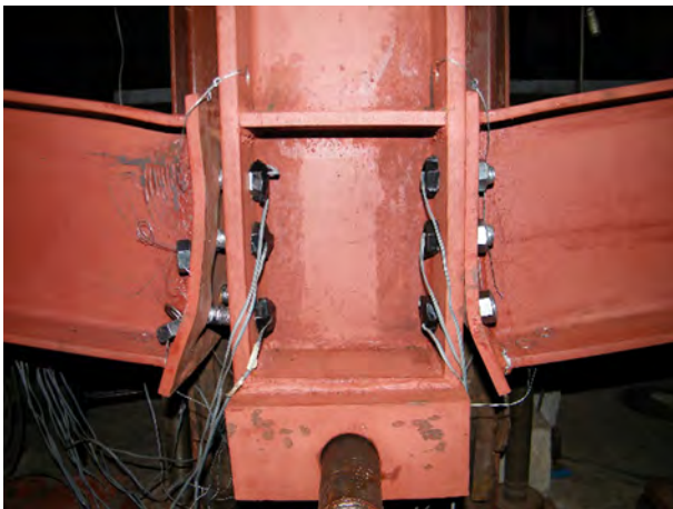
Fig. 5. Failure of a beam-column joint in a specimen tested by Yang and Tan [160]. Photo by courtesy of Bo Yang (Chongqing University).
