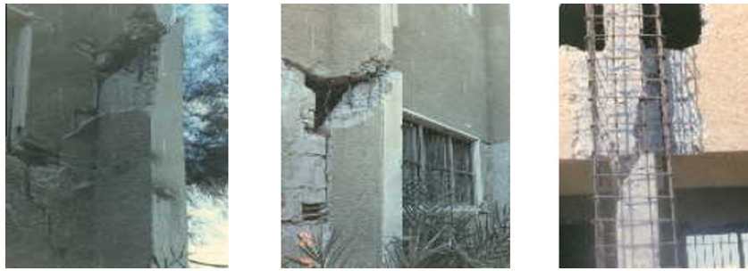
Fig. 2 School buildings at Fayoum, Egypt, after 1992 earthquake [12].
