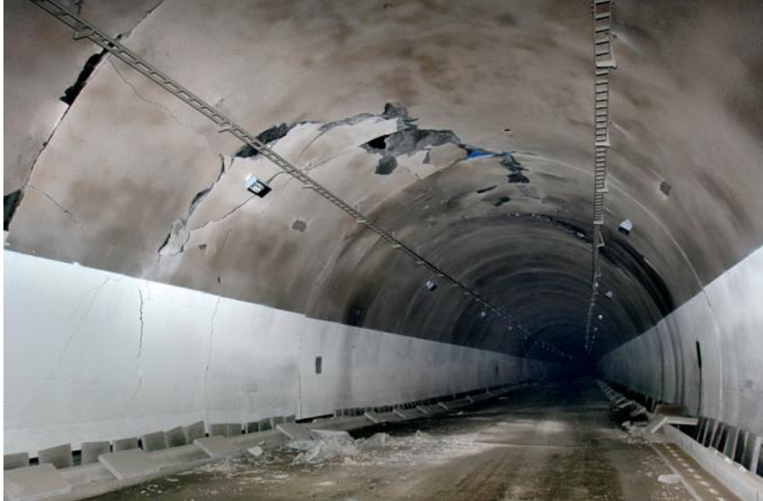
Fig. 7 Longdongzi Tunnel after the Wenchuan earthquake. This tunnel located near Dujiangyan City. It was damaged but didn't collapse in Wenchuan earthquake. Actually none of the tunnels in the area were found to have collapsed during the Wenchuan earthquake's powerful shaking motions. Since few fault lines dissected a tunnel in this earthquake, almost all of the tunnels in the area (even in the intensity X degree areas) had suffered no or only slight damages during the earthquake event (Lu Ming).
