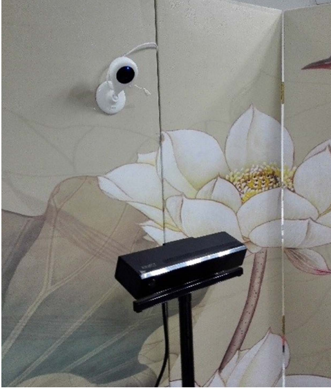
Figure 20.4 An IP camera has been installed to capture the interactions between players and the “affective” objects.
