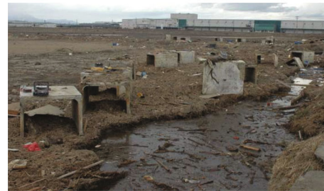
(b) Damage due to liquefaction and tsunami
