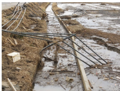
(a) Damage due to tsunami only
