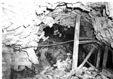
Fig. 5. 1957 burst site in the main slope at the Sunnyside Mine [7].
