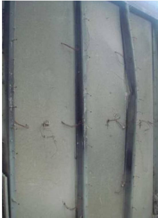
Figure 4. Cold-formed steel frame after fire [12].
