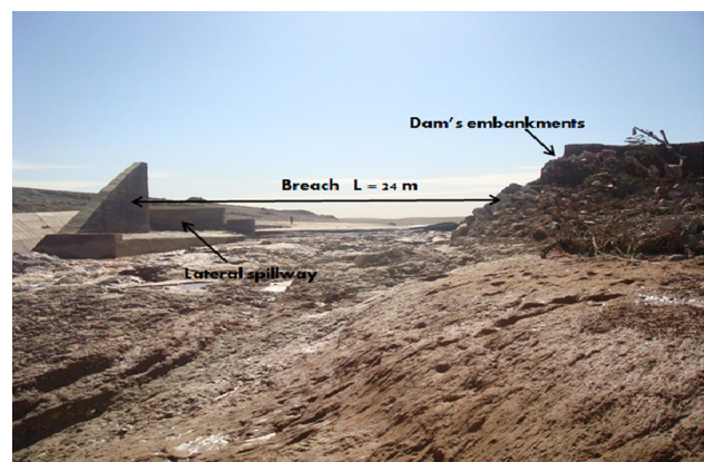
Fig. 2 Damages recorded in spillway's zone—October 2005
