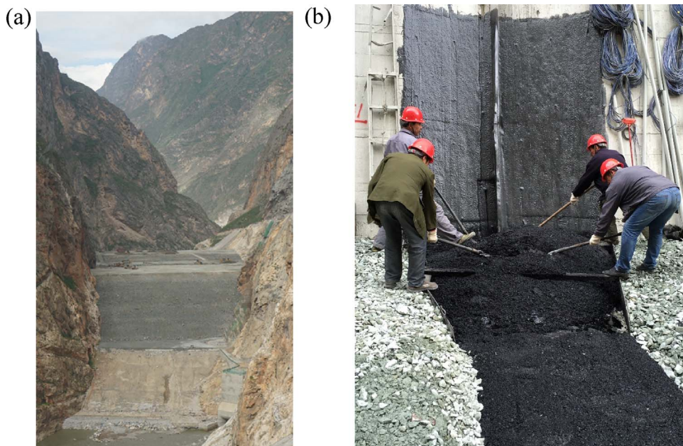
Fig. 1. (a) The 174-m high Quxue Dam under construction; (b) asphalt core-plinth connection on the dam left abutment with a slope of 1 V: 0.33H (72°).
