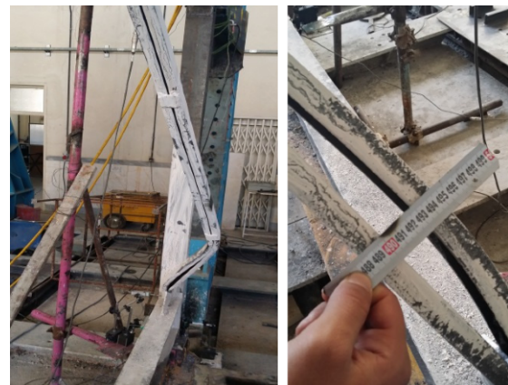
Figure 6. Large out-of-plane deformation of brace in Test 1.
