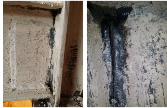
Figure 11. crack in connection of beam to column in test 3.
