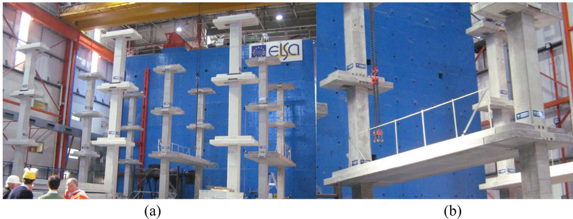
Fig. 8. Full-scale prototype: (a) monolithic columns with cross-shaped corbel for the support of the shallow hollow core beam and floor members, (b) beam in phase of assemblage.
