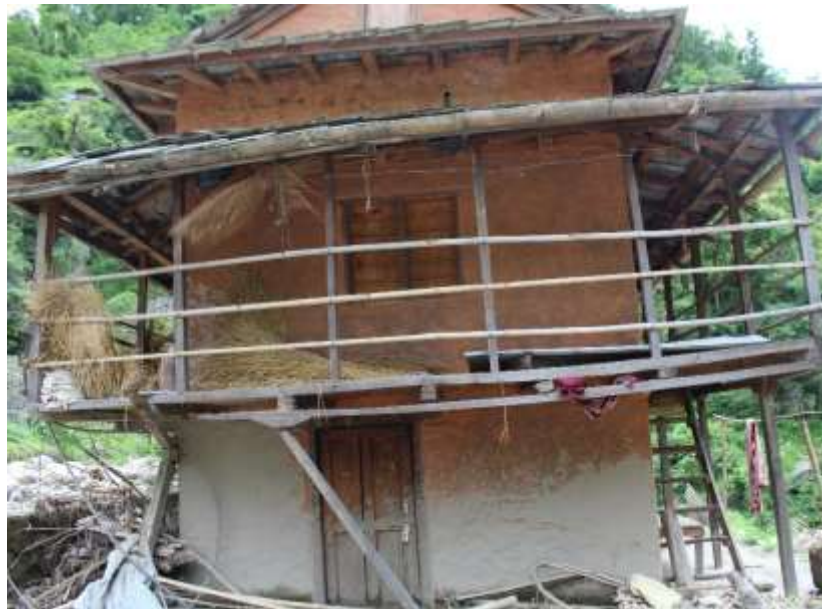
Fig. 8 The flood unaffected but earthquake damaged (minor) vernacular building
