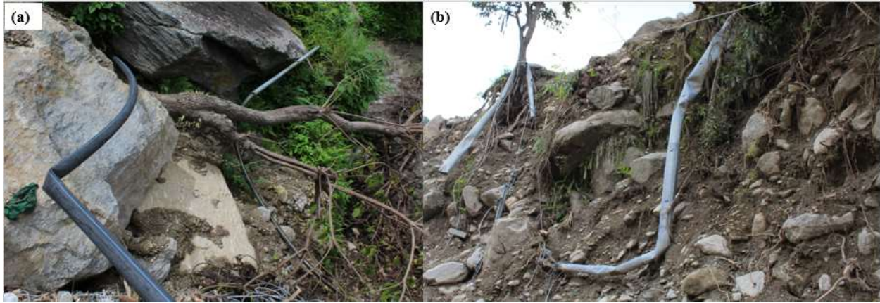
Fig. 6 a) Damage water supply pipeline and b) damaged to the electrical poles
