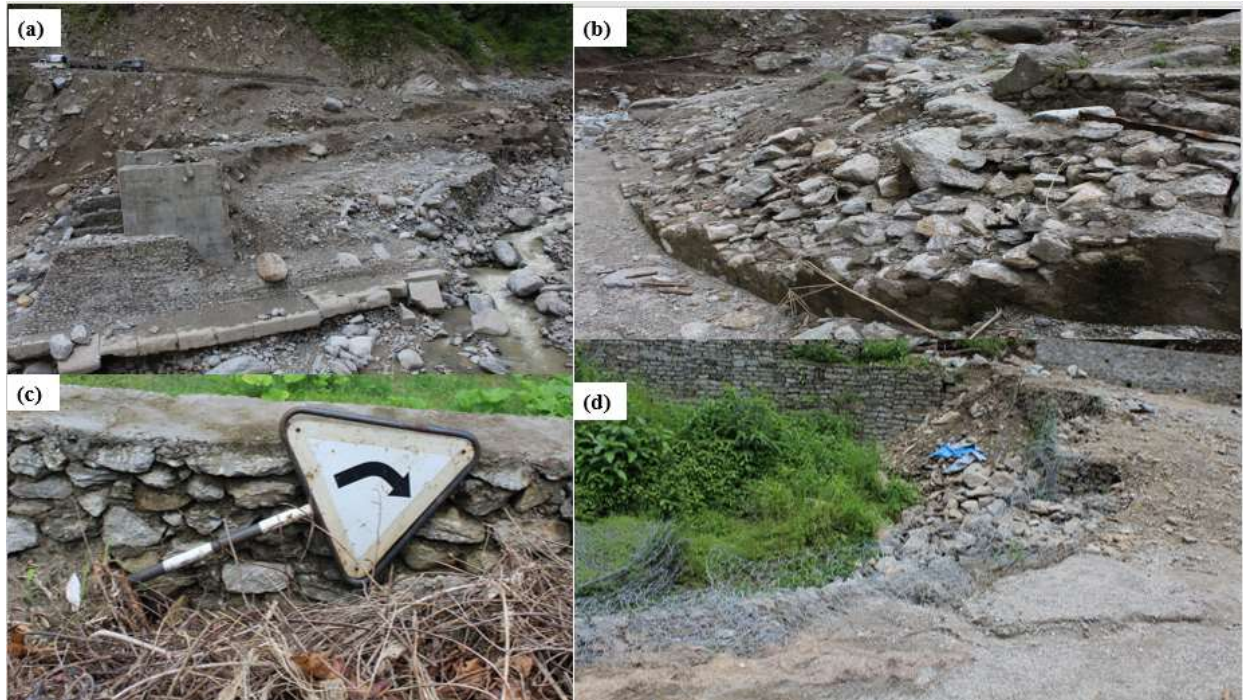
Fig. 5 a) Road damage due to flash flood; ~2 km long stretch was washed away with no indication of road alignment; b) exposed subgrade of the road; c) damaged sign post along the road; and d) damage to the gabion wall
