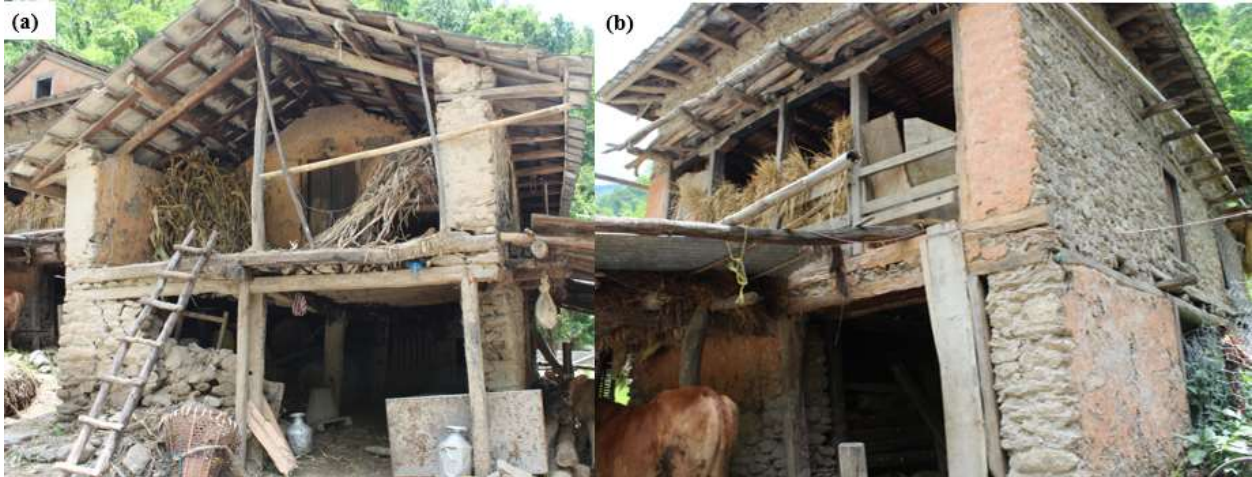
Fig. 7 a) severe damage and b) major damage to vernacular buildings
