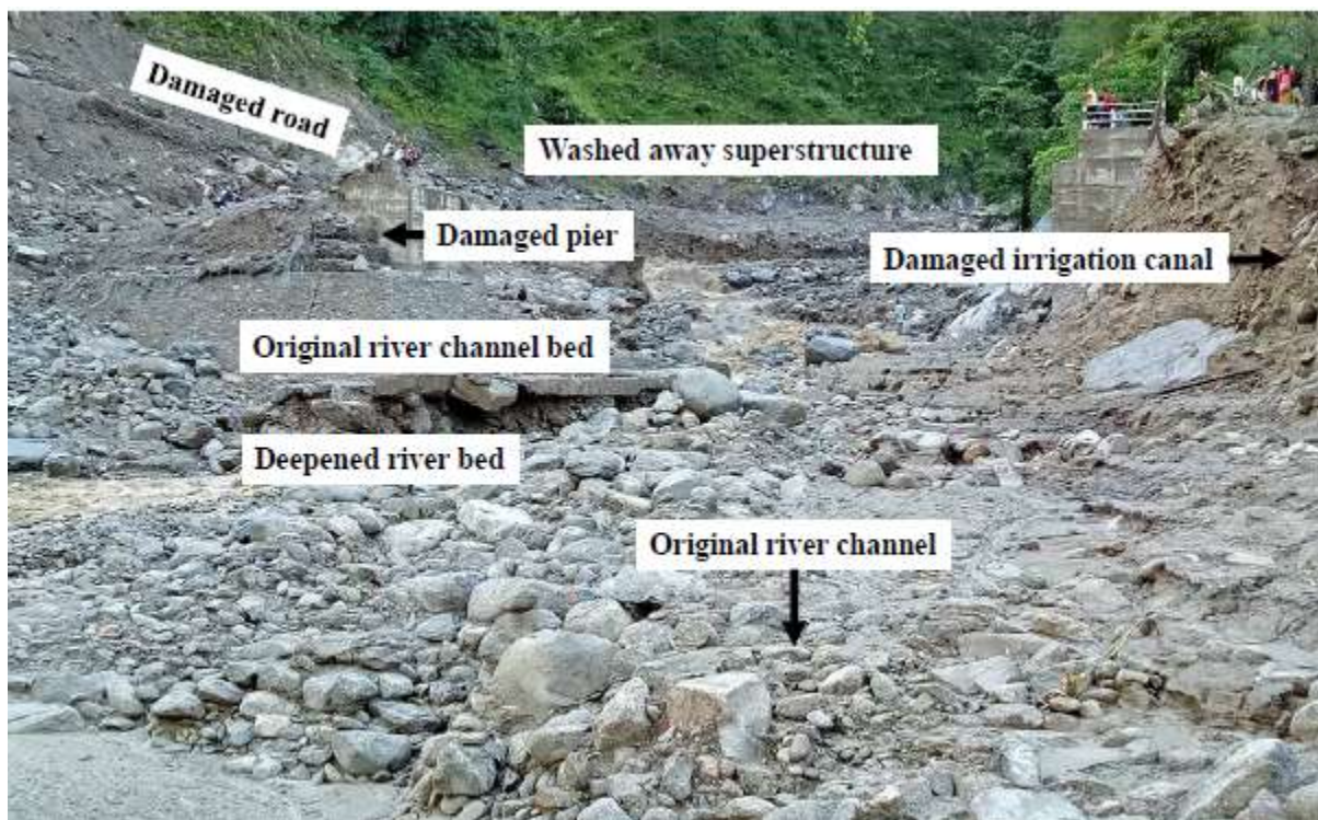
Fig. 3 Debris flood from the stream due to flash flood in the bridge site
