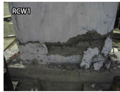
Transverse crack at the bottom
