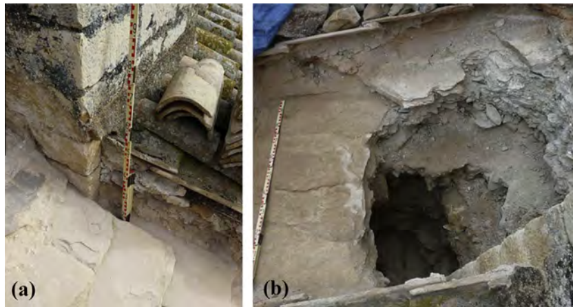
Fig. 4. Infill of the barrel vault: (a) upper part of clay tiles, sand and stone tiles and (b) lower part of poor quality filling materials [32].
