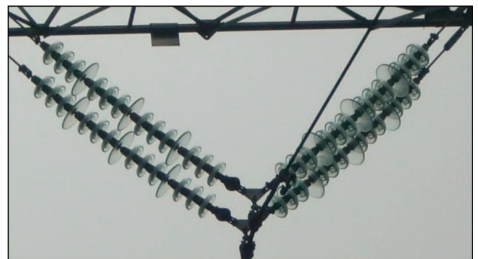
Figure 3. Changing insulator orientation at 220 kV (Guanlang Line in Guangdong).
