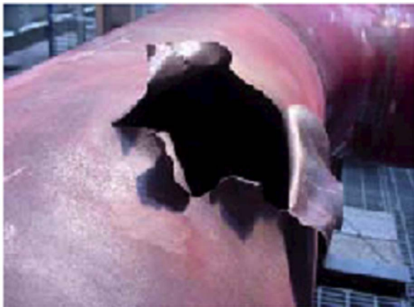
Fig. 8 Example of pressure blowout occurring at thermal power plant piping
