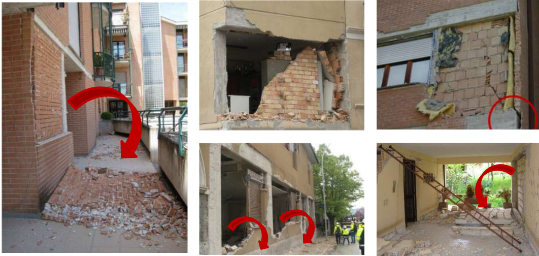
Fig. 1. IM walls out-of-plane collapses when subjected to earthquakes.
