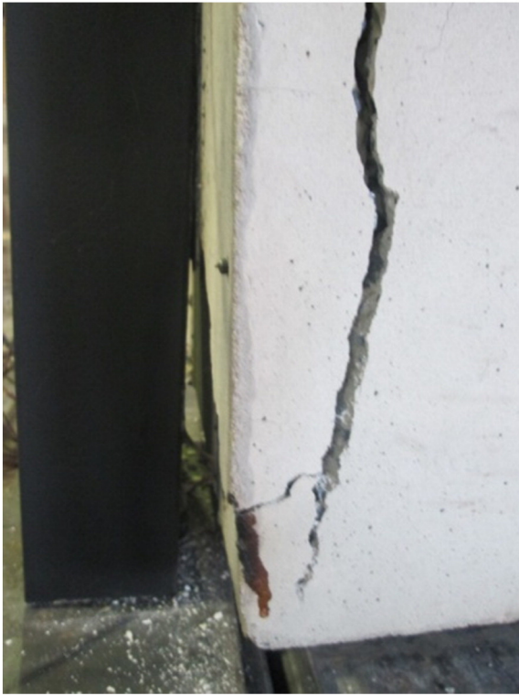
Fig. 10. Failure mode of Blind Bolt 1 connector specimens post-fire.
