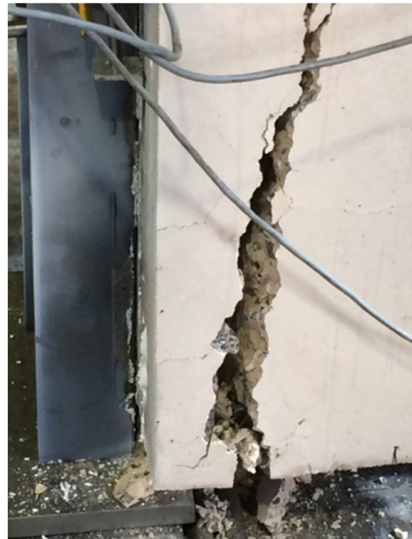
Fig. 14. Failure mode of Blind Bolt 2 connector specimens post-fire.
