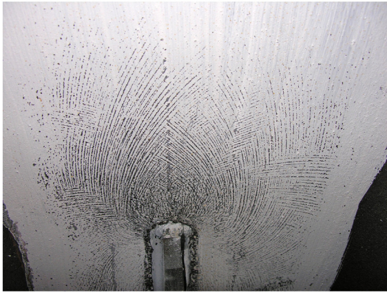
Fig. 6. Column Web Lüders' Lines at the Compression Edge of the Plate.
