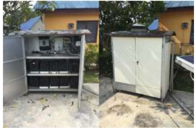
Fig. 21. Photo of battery bank room.
