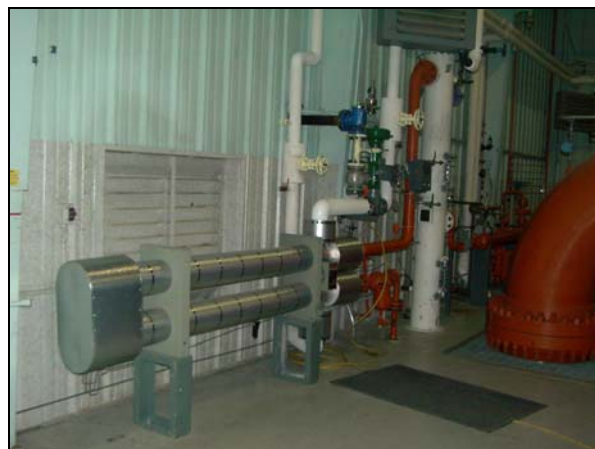
Heat Exchanger (Left) Coalescing Filter (Right)
