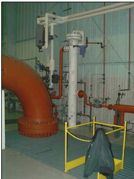
Coalescing Filter (Centre) 1 st Cut Regulator Filter/Separator (Right)
