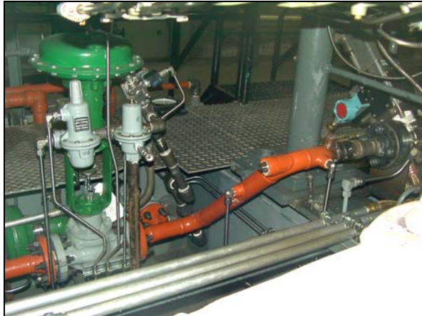
High Speed Shut-off Valve (Left) Fuel Modulating Valve (Right)
