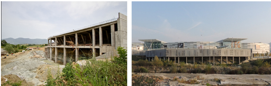
Fig. 5. Photo of completed frames (left) and present state of the structure (right).
