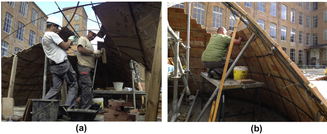
Fig. 2. Building Brick-topia's first layer of bricks: (a) applying fast-setting cement and placing the brick, (b) cleaning the joint. © Manuel de Lózar and Paula López Barba.
