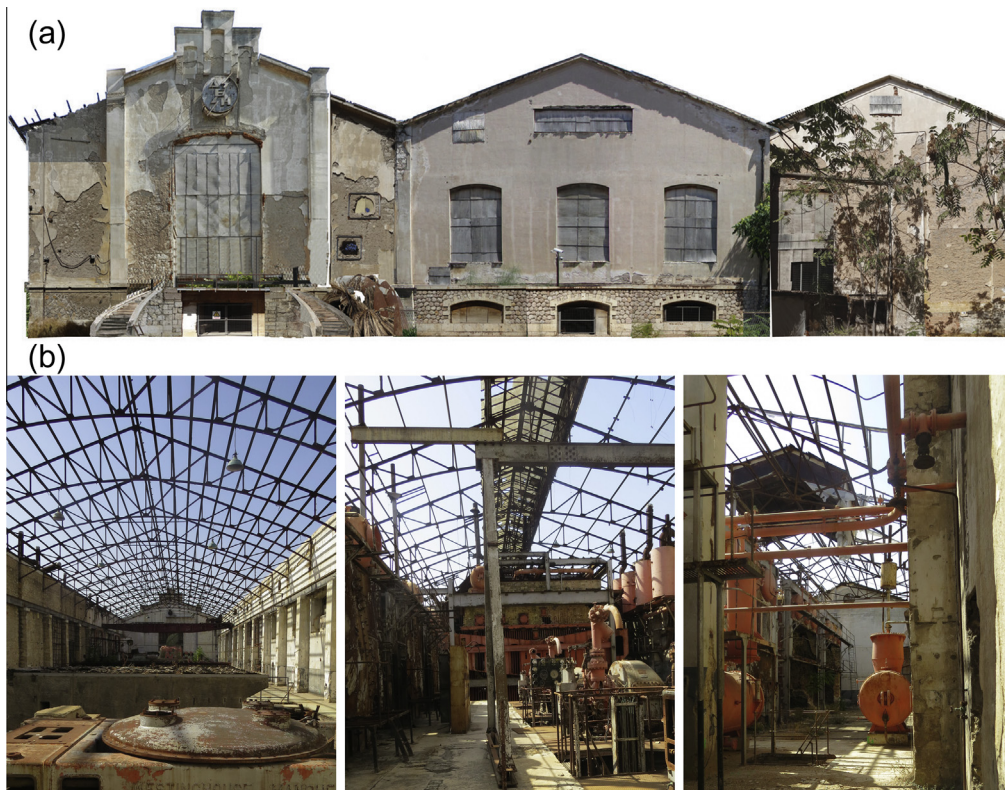
Fig. 1. Exterior (a) and (b) Interior of buildings A, B and C2 on the mezzanine level.
