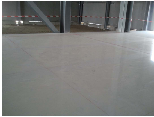
Fig. 13. Photo of a treatment by overtopping with self-levelling and high resistance resins (Floor No. 3)
