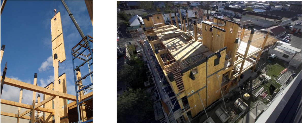
Fig. 4. Photos taken during construction and installation of LVL post-tensioned and coupled shear panels.
