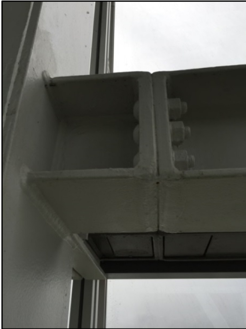
Fig. 5. Typical stub detail for connecting an open section beam to a box section column.
