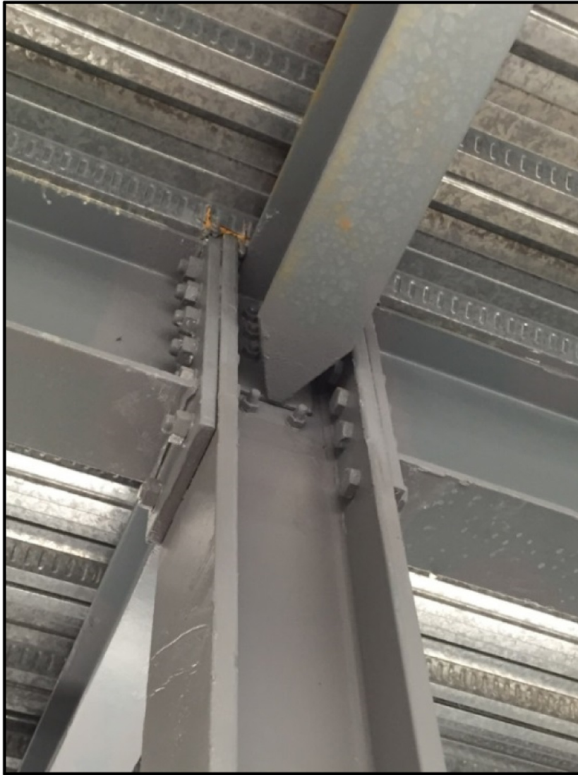
Fig. 10. Typical crowded connection where a Draftsman/Detailers input or use of 3D BIM may be invaluable.
