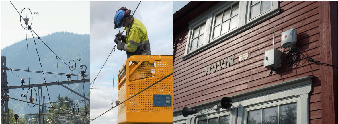
Fig. 6. Mounted monitoring system at the Hovin station: left—sensors; middle—mounting of a sensor; right—master unit and wireless wide-area network antenna. Photo: NTNU/Petter Nàvik.
