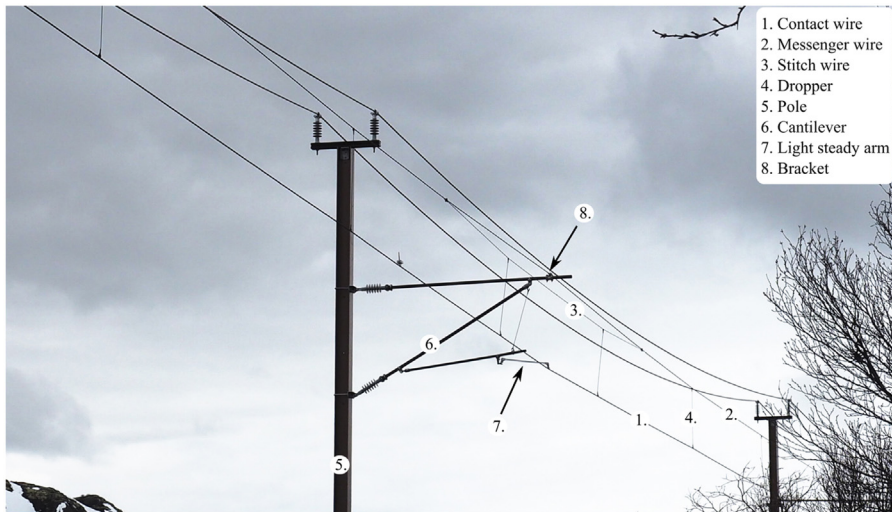
Fig. 3. Presentation of important structural components of railway catenary systems. Photo: NTNU/Petter Nāvik [10].
