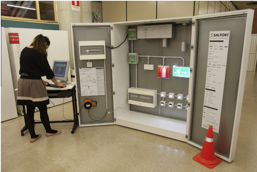
Fig. 2. Emergency lighting cabinet.
