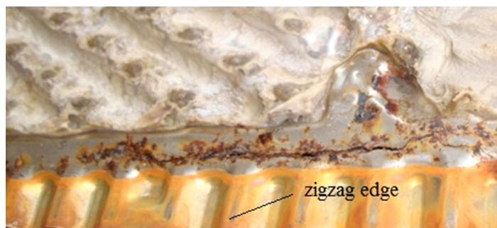
Fig. 3. Presence of cracks and pits on gasket sitting groove.
