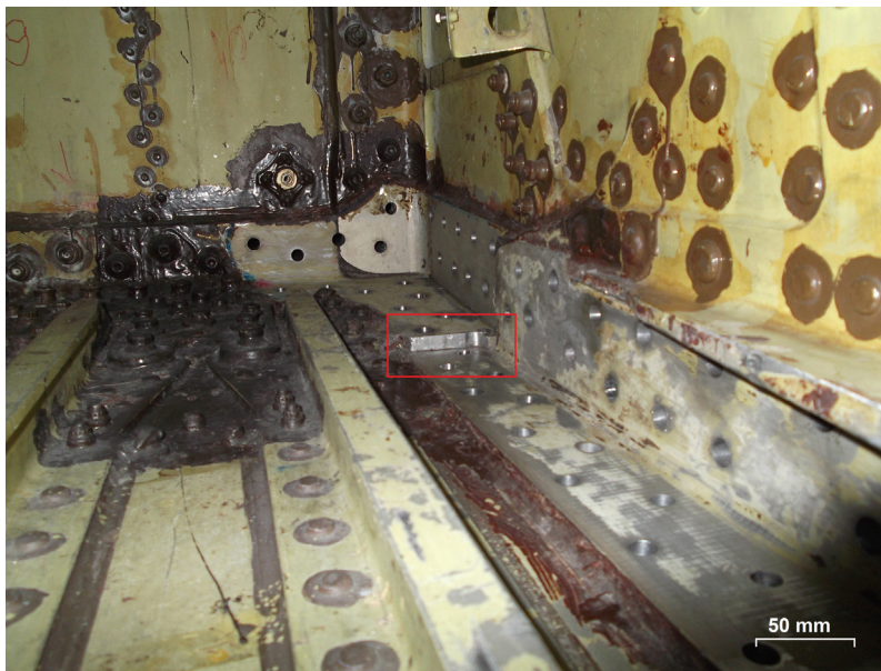
Fig. 4. Installation place of the angle at the corner of center box (step shaped geometry is highlighted in a red rectangular). (For interpretation of the references to color in this figure legend, the reader is referred to the web version of this article.)
