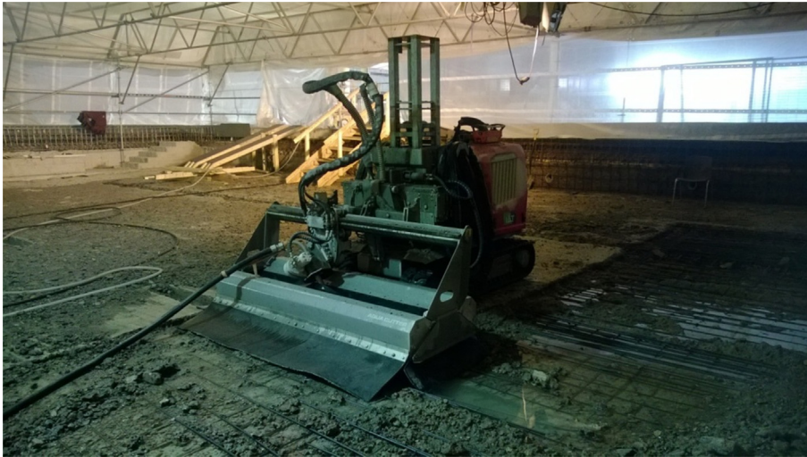
Fig. 4. The working width of the high-pressure water-jet cutter was 2 m. Concrete was removed under a temporary shield.
