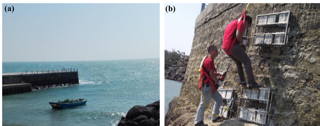
Fig. 3. Construction photograph of marine field concrete samples in Zhanjiang, Guangdong, China. (a) Naozhou island in Zhanjiang, (b) field construction after falling tide.
