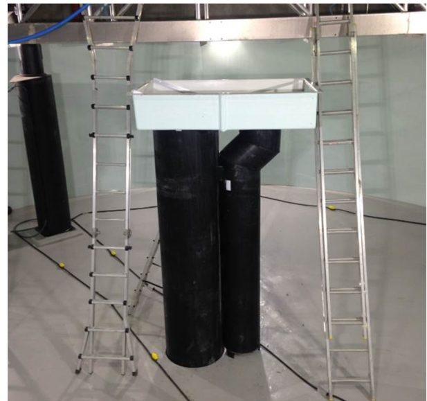
Fig. 6. Large drain structures used to rapidly remove dead or moribund fish from the tank center provide a huge benefit to the tank operator but also impact culture volume hydraulics.
