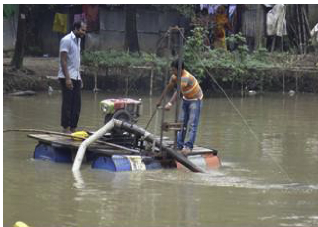
Fig. 4. Photograph of operation of sludge remover.
