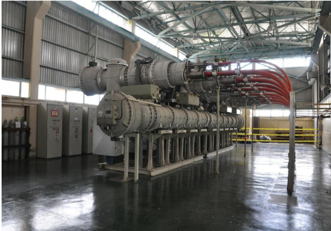
Fig. 1. High voltage switchgears.
