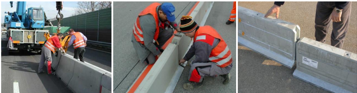
FIGURE 5/6/7 Installing Concrete Barriers – New Jersey type barriers with heavy equipment (l), slim-type barriers with screws (m), tight-fitting superlight barriers without any tools (r)
