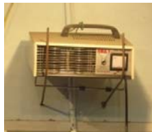
(c) Room Heater
