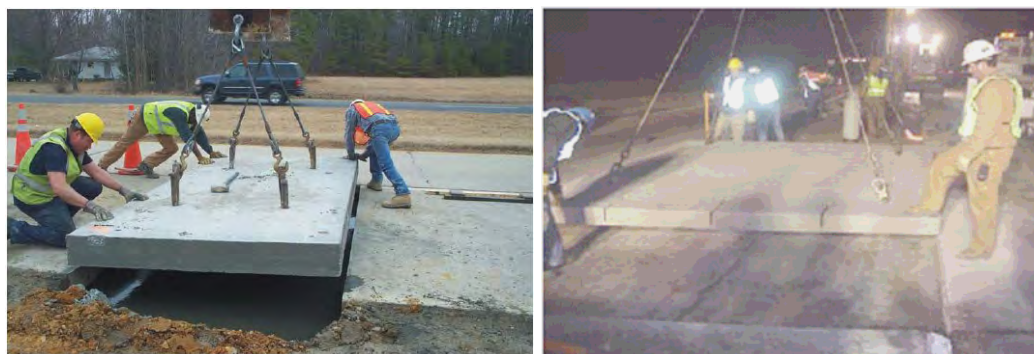
Figure 6. Precast concrete panels for experimental slab replacement in Virginia (17) and in Colorado (18).
