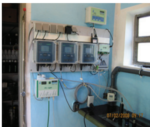
Fig. 2. The interior of the automatic station Beli Brod.
