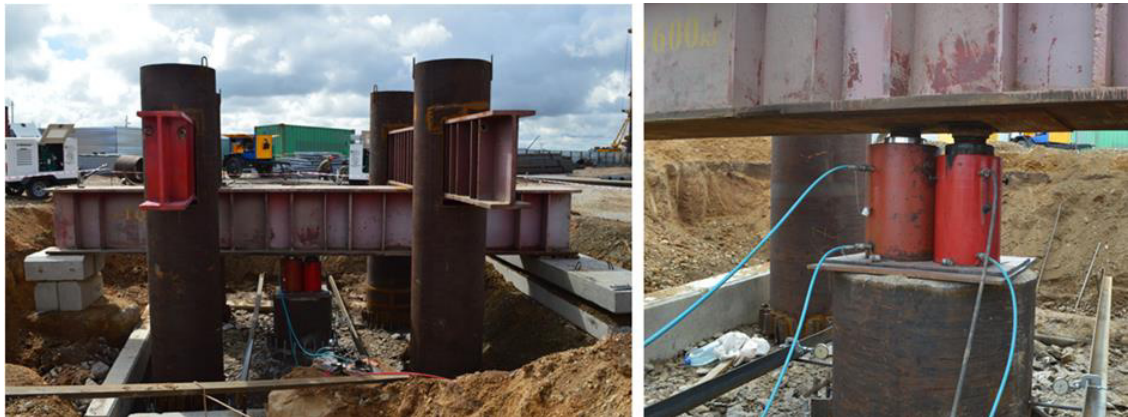
Fig. 4. Static Load Test of bored piles in construction site New Railway Station, Astana.
