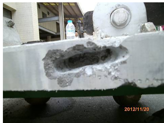
Fig. 18. Corrosion in Tanduliao sluice gate.
