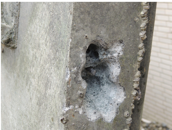
Fig. 17. Corrosion in Houanliao sluice gate.
