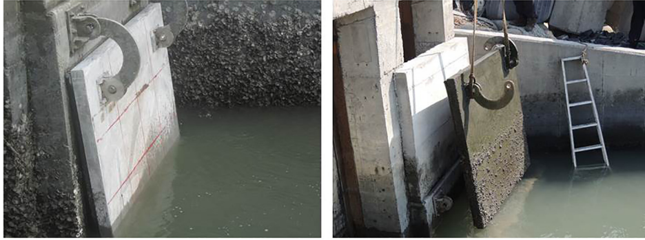
Fig. 13. The appearance of the Houanliao sluice gate (after 12 months of field testing).
