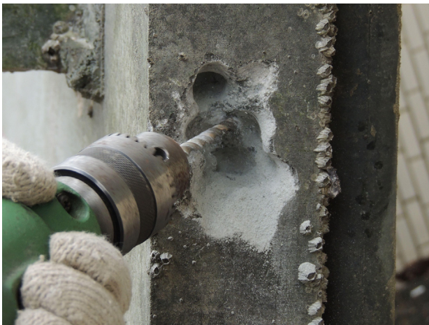
Fig. 16. Drilling one edge of sluice gate to assess the corrosion of rebars and wire meshes.
