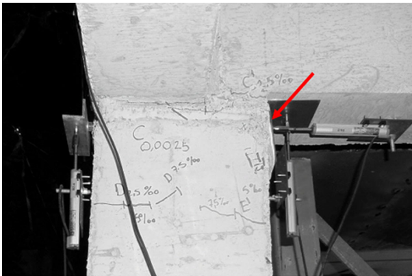
Fig. 16 Cover spalling at 2.50 % drift ratio in column S11
