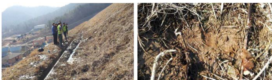
Fig. 8. HD dam: leakage and wet zones observed on the downstream surface.
